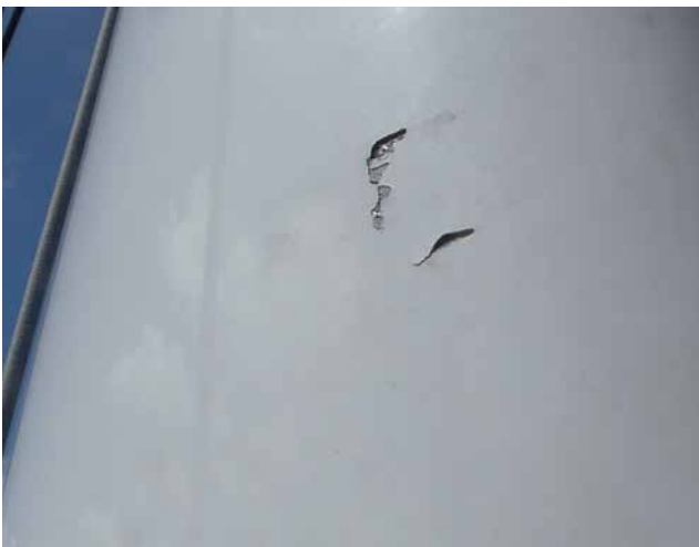
Damage can appear minor
