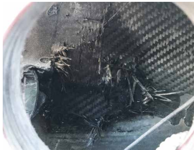
The endoscope reveals delamination
